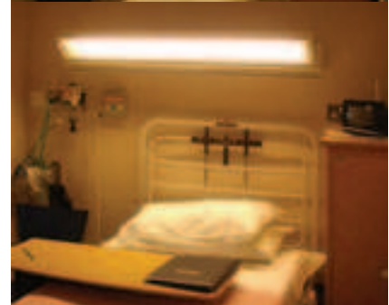
Figure 4.62 Traditional bedhead lighting is flexible for uplighting only (top) or for task lighting and medical examinations (above)
